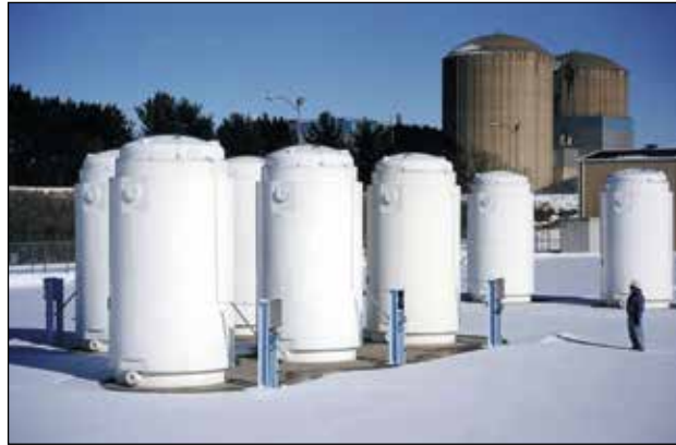
TN-40 Dry Storage Cask
